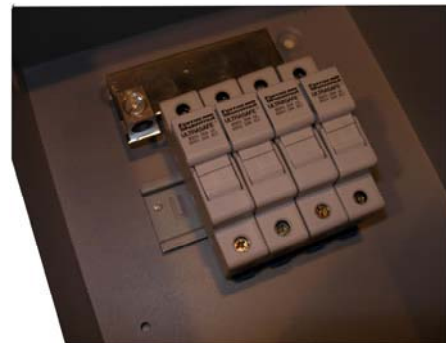
Fuse holders in enclosure
