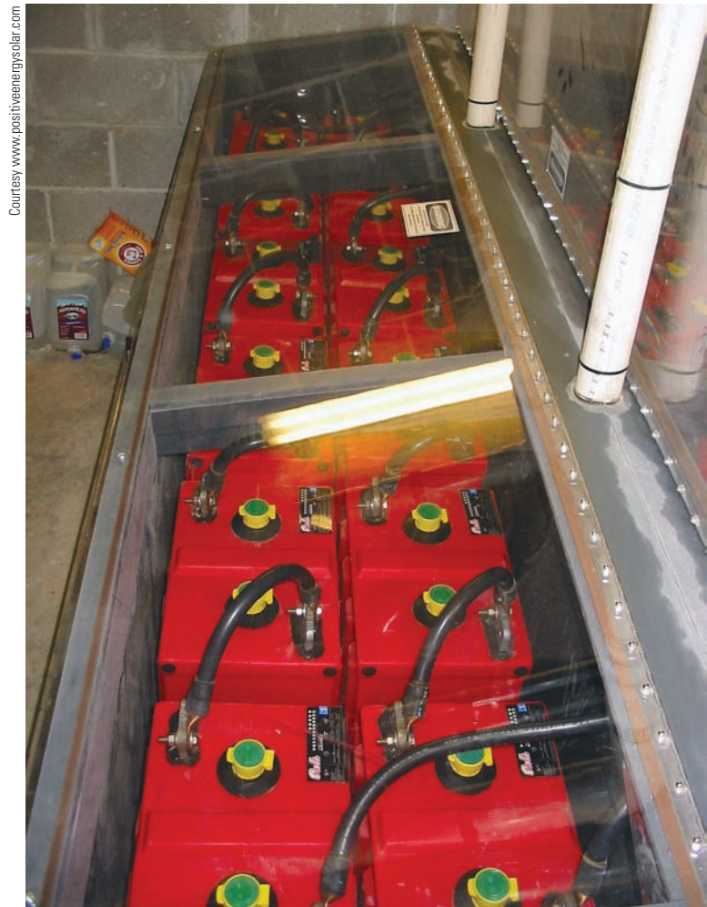
A well-constructed, site-built battery enclosure.
